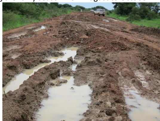
E. Road damaged before Maper (40km, after 3 dry days)
