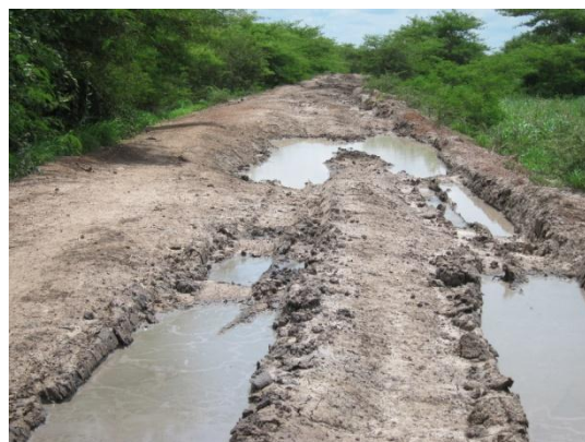
R. Mir Mir-Tharjath road damaged (11 July 2013)
