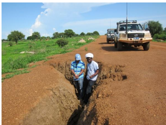
C. Road erosion at Gongor culvert
