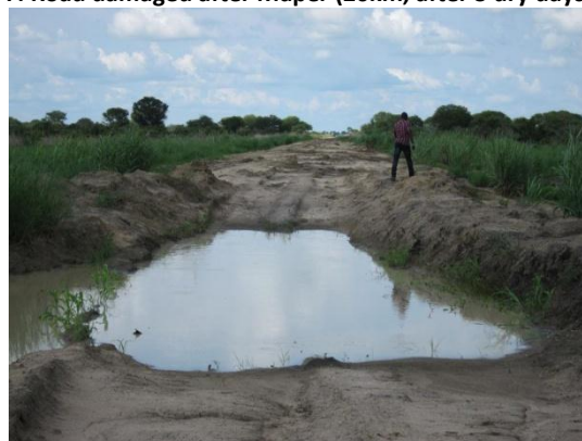
H. Road damaged after Madol (after 3 dry days)
