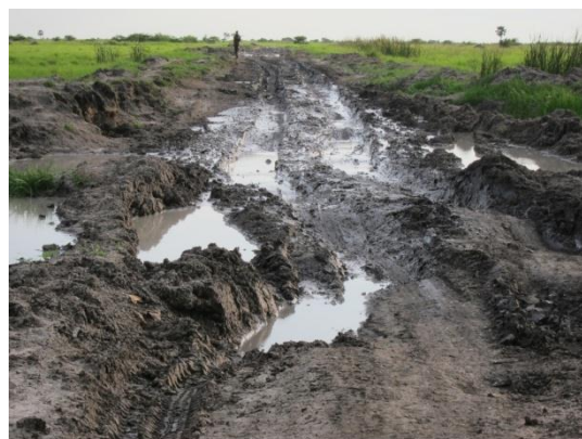
J. Road damaged before Mayendit (8 July 2013)
