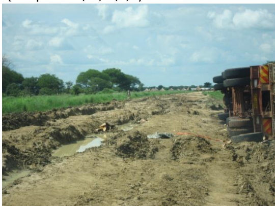
G. Road damaged before Madol (after 3 dry days)
