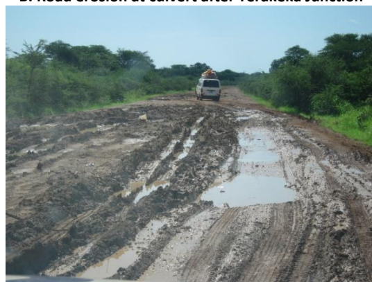
D. Terakeka-Awerial road is in bad condition
