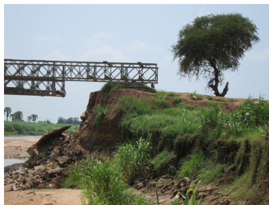
AG: Luri Bridge, damaged on 18 July 2013(after; close-up)
