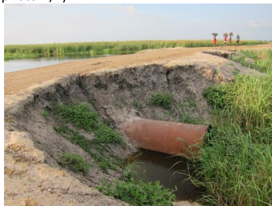
L. Mayendit culvert road eroded (8 July 2013)
