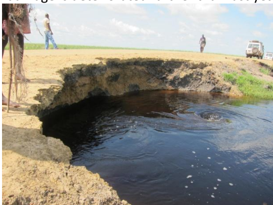
K. Mayendit culvert road eroded (2 Sep 2012)
