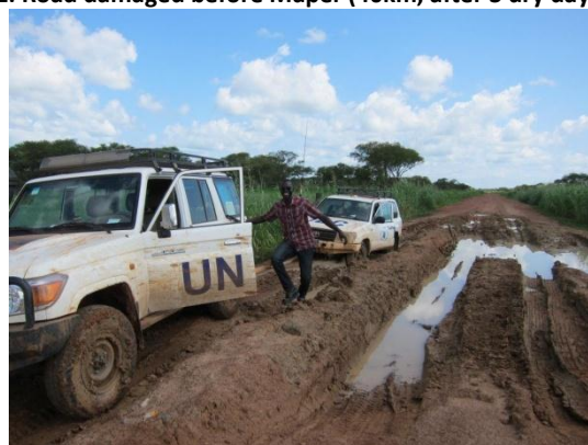
F. Road damaged after Maper (20km, after 3 dry days)
