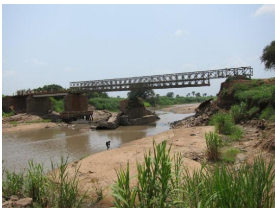
AF: Luri Bridge, damaged on 18 July 2013(after)
