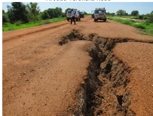
B. Road erosion at culvert after Terakeka Junction
