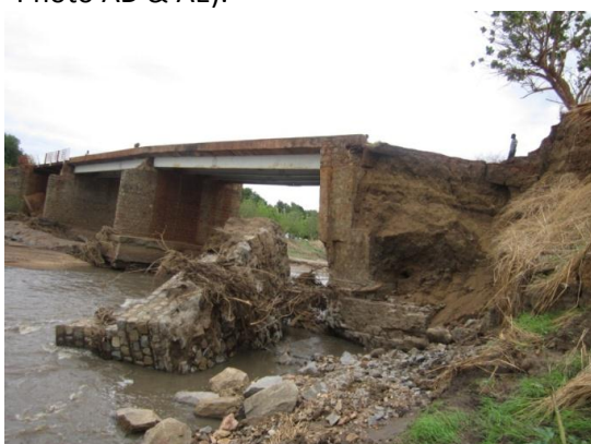
AD: Luri Bridge, damaged on 27 April 2012(before)
